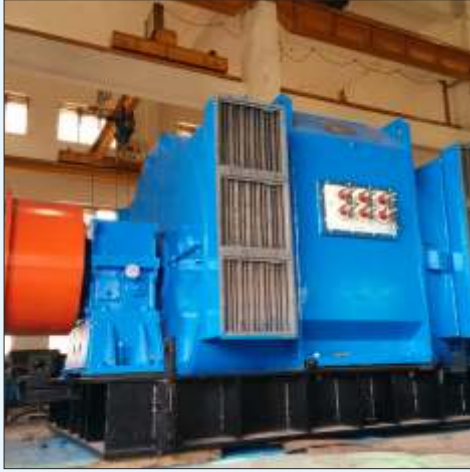
7.5MVA,6.6 KV, Alternator Post Overhauling
