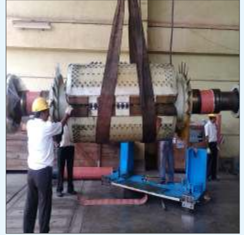
35MVA, Alternator Rotor Threading Out
