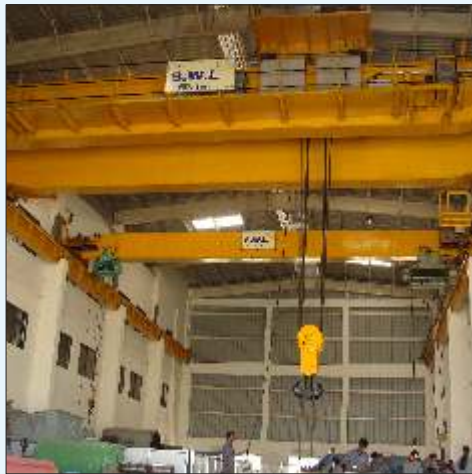
65T, EOT Crane
