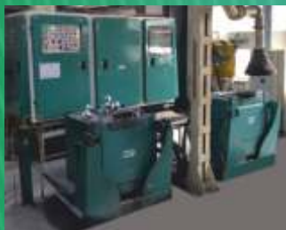
Induction Melting Furnace 100kg/Hr. capacity
